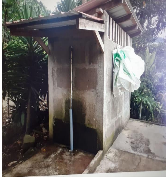
Shower installation in a precarious situation. It lacks walls and a door to guarantee privacy.
